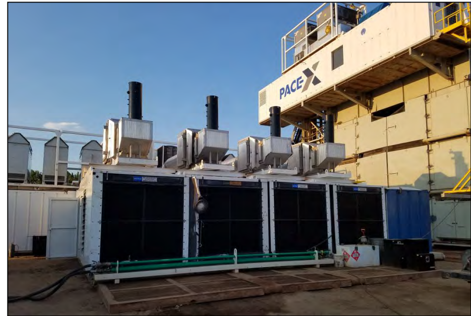
Each diesel engine equipped with SCR+ASC system, above engine
